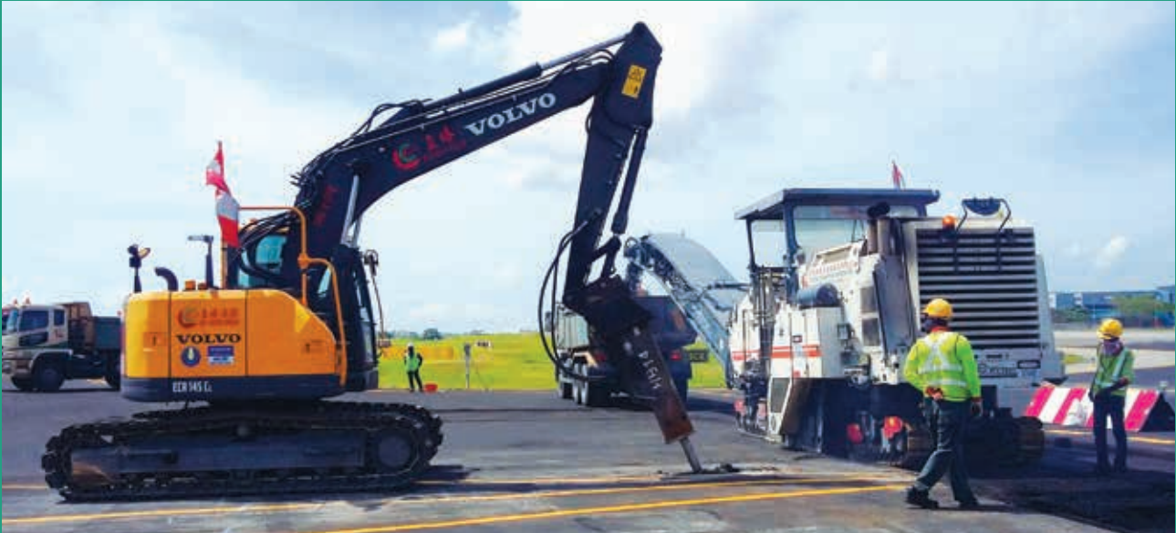
◆ Milling and patching of asphalt premix for airport taxiway and installation of air field lighting
